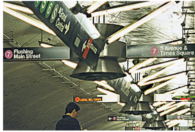
Functional stainless steel ceiling sculpture on 7 platform incorporating lighting, signage, LED, and fan system
